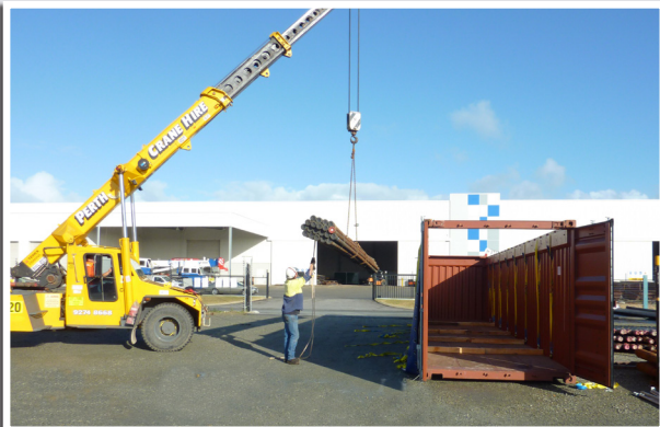
A crane is used to lift a bore casings into the sea container.
