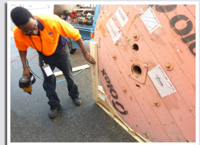
One of the vertical timber dunnage pieces being attached to the pallet and the cable drum.
